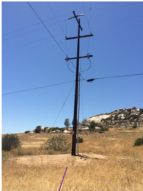
Photograph 2: View of proposed temporary workspace area at Structure No. D193 and overland travel entrance, facing west.
